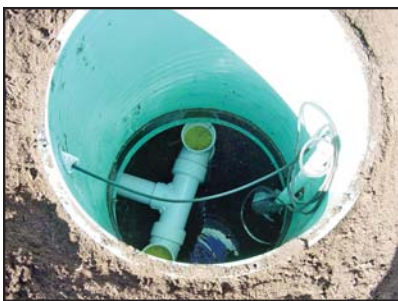
The middle manhole of the Dyno2 unit shows the high-water alarm float and the top of the yellow brush-like filters.
